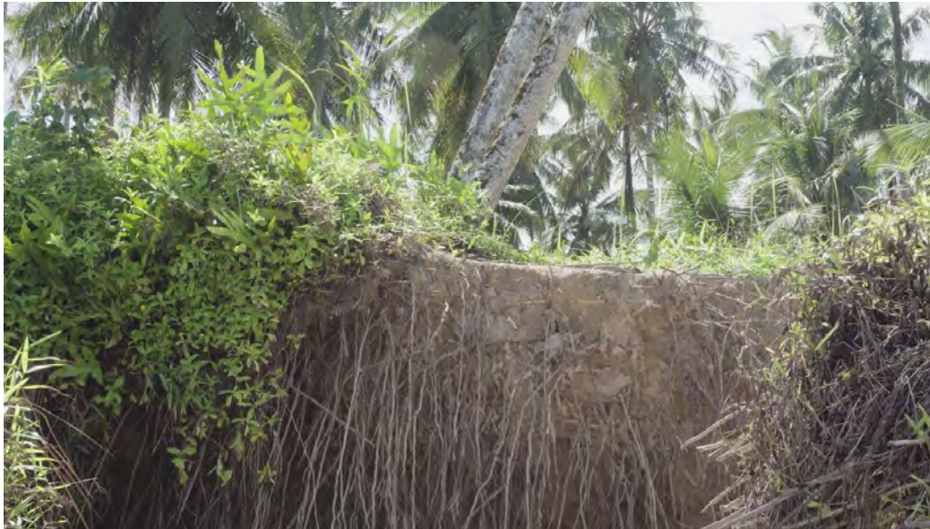
Figure 31: Sand erosion on the banks leading onto the mainland, due to constant mining
