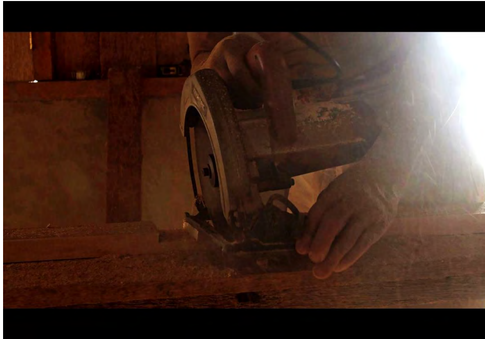
Figure 34: A still from the 2018 archive footage – construction work on the new school building
